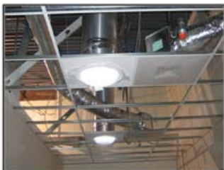
The new building will feature over 100 Solatubes which direct natural light into interior spaces
