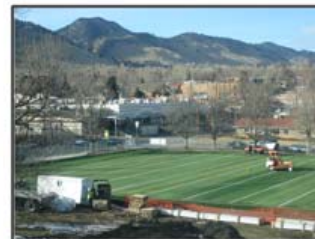
Geothermal wells, which provide energy efficient heating and cooling for the building, have been installed under the synthetic field
