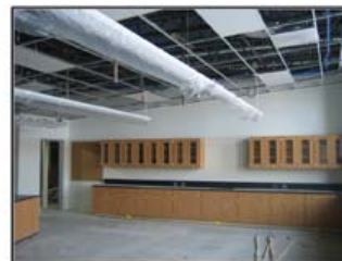
Classrooms on the north side of the school take advantage of daylighting opportunities
